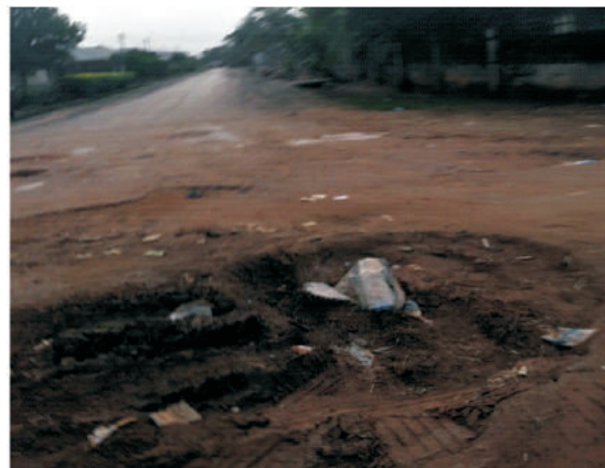
Plate 23: Estate road eroded by rainwater
