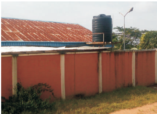
Plate 6: Overhead tank for water storage
