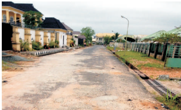
Plate 12: Road showing patched up areas
