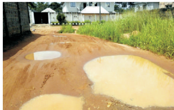
Plate 31: Potholes on the road
