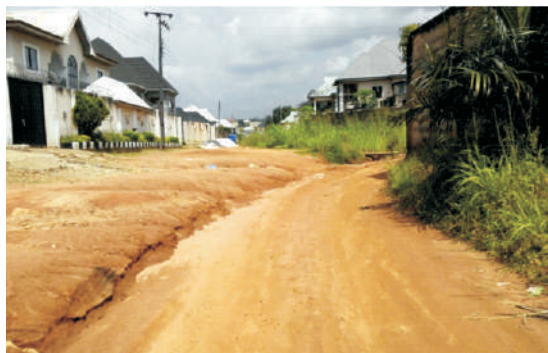
Plate 30: Road badly eroded by water
