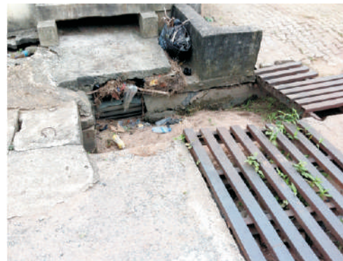
Plate 13: Blocked and broken drain
