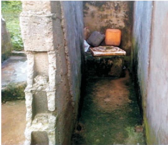
Figure 5: An abandoned toilet
